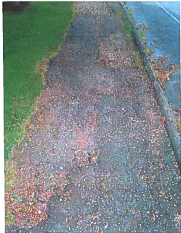
Missing pavement on Wadsworth St. sidewalk
