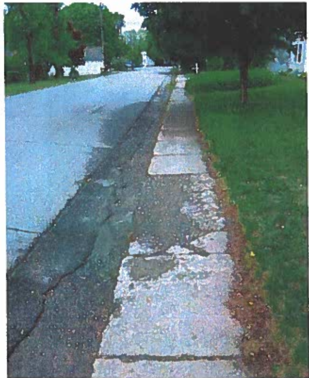
Broken and failing sidewalk by house #20
