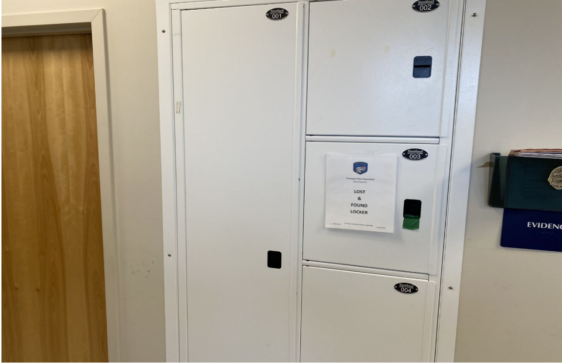
Pass-through evidence storage
